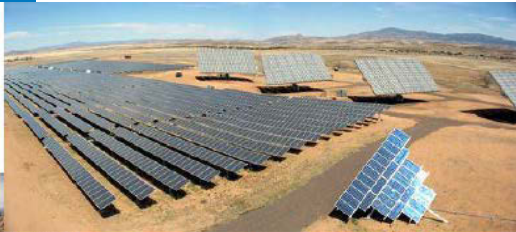
Arizona Public Service, Prescott, Arizona Photo from Arizona Public Service
