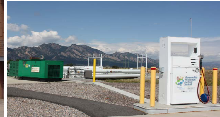
Distributed Energy Resources Test Facility (DERTF)
