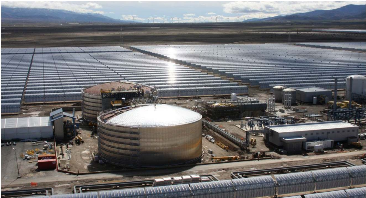
Figure 2. An oil-HTF parabolic trough plant with molten-salt TES tanks under construction. Photo courtesy Solar Millennium AG
