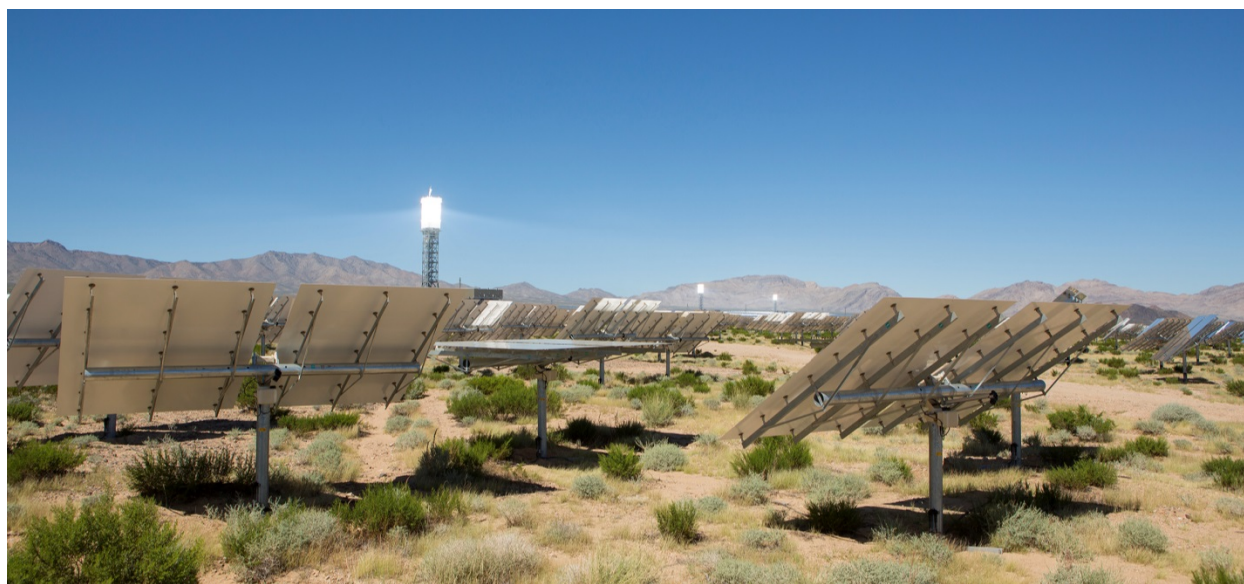
Figure 5. LH-2.2 heliostats at Ivanpah.
