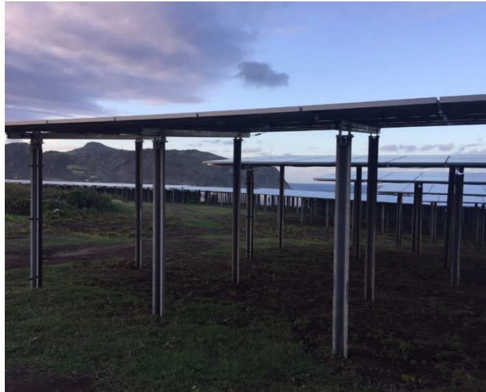
Figure 7. Novel mounting height of solar panels at Statia solar and energy park
