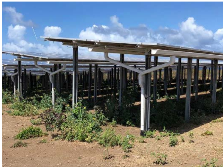
Figure 8. Rainwater-harvesting gutters mounted to PV array
