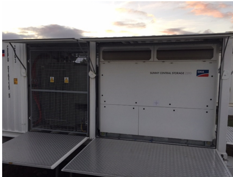
Figure 3. Grid-forming battery inverter
