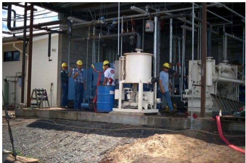
Figure 5. Biomass gasifier that uses residue from the nearby sugarcane mill—Maui, Hawaii
