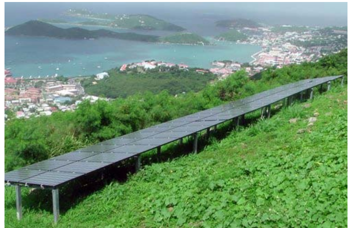
Figure 3. 10 kW PV system installed on St. Thomas, U.S. Virgin Islands PIX 19568
