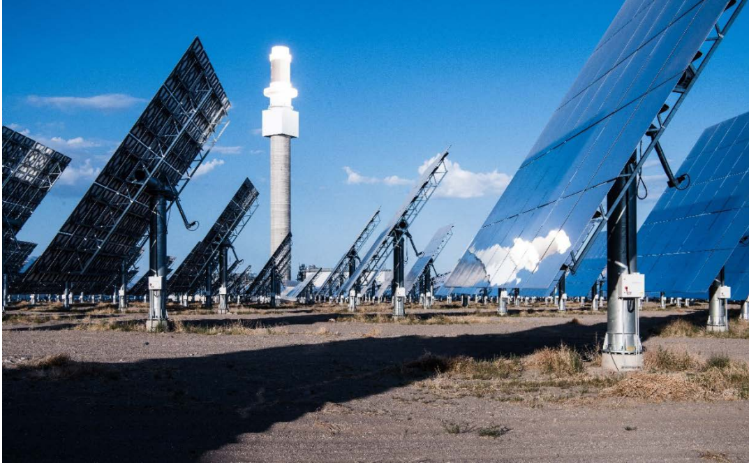
Figure 2. Power tower concentrating solar-thermal power systems such as this one use focused mirrors, called heliostats, to reflect sunlight onto a receiver on top of a tower. Each heliostat uses a two-axis tracking system to focus the sun on the power tower receiver.
