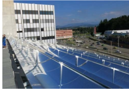
Figure 5. CSP PTCs used for generating heat at the Cremo SA milk processing centre
