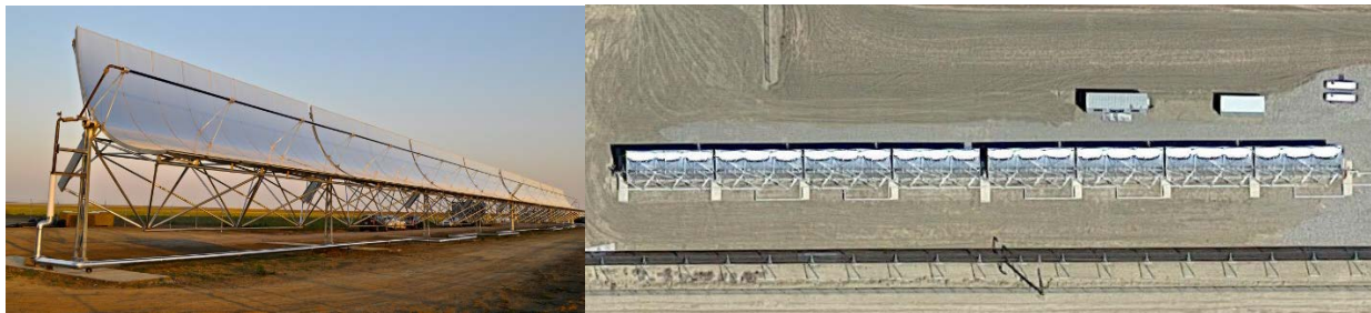
Figure 32. SkyTrough CSP collector at the Panoche desalination pilot plant 140
