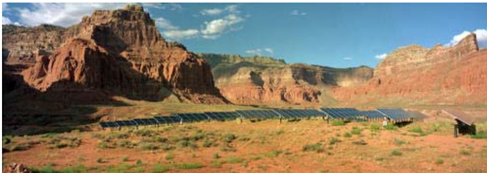
Figure F- 3. This 160 kW PV system in Utah is similar in size and type to the system considered here.
