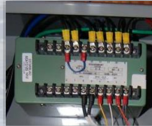
Power, VA, Volts transducer (external CT's)
