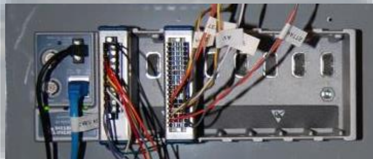
Data Acquisition (chassis and modules)
