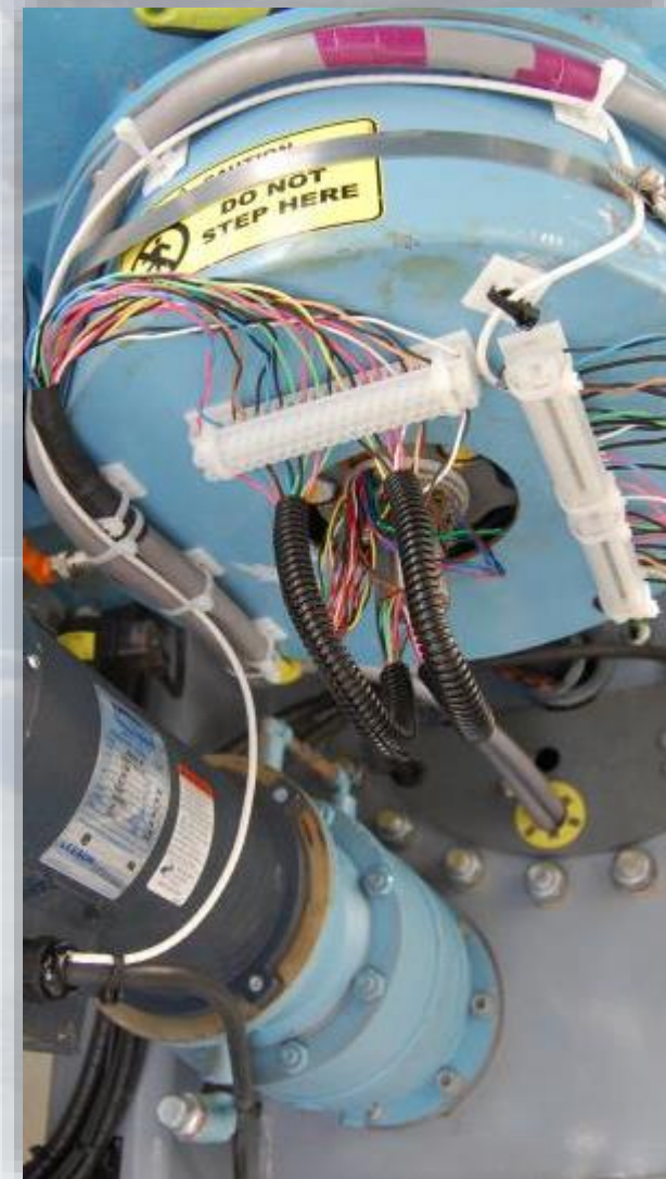
Slipring transmitting data from rotor through main shaft
