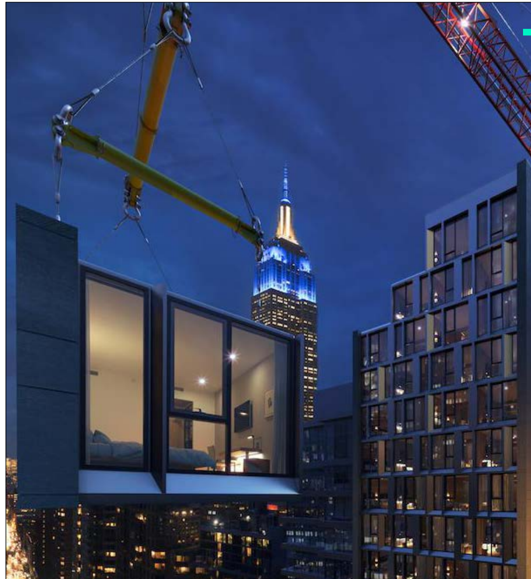
FIGURE 4 A crane lifts a volumetric modular hotel room unit onto the AC Hotel New York NoMad at 842 Sixth Avenue. Source: Skystone.
