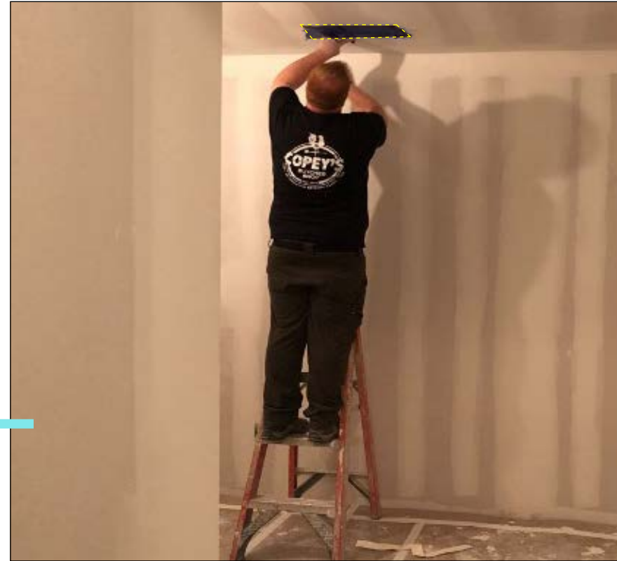
FIGURE 24 Prep stage prior to ionized sealing, showing sealing supply register. Source: Photo documentation of VBC Pilot 2.
