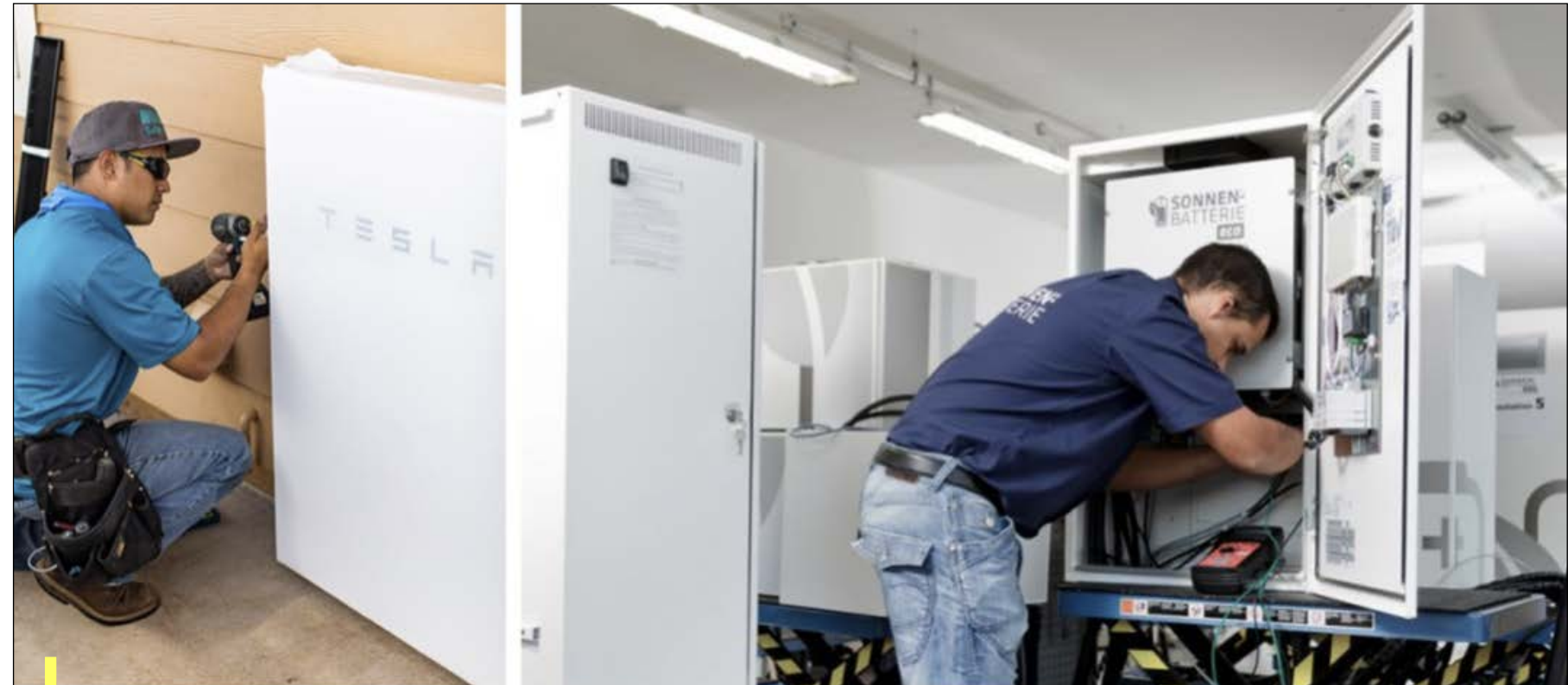
FIGURE 41 Ease of installation and maintenance of small, distributed home batteries. Tesla Powerwall Certified Installer (left). Source: Tesla Inc., sonnen Inc.'s U.S. factory (right). Source: sonnen Inc.
