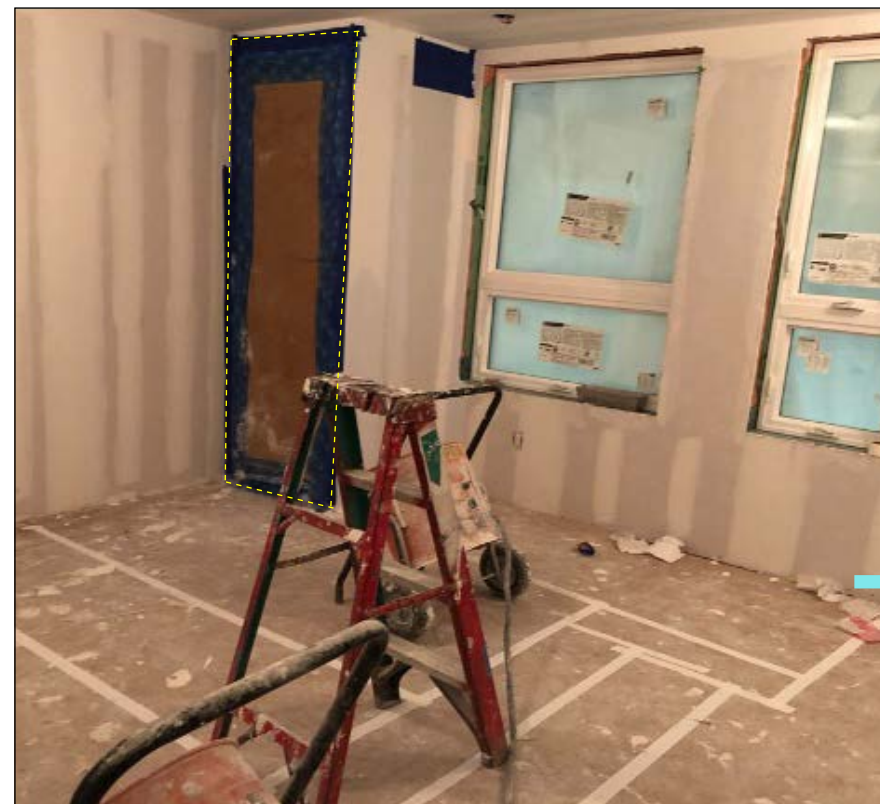
FIGURE 25 Prep stage prior to ionized sealing, showing covering and taping utility room. Source: Photo documentation of VBC Pilot 2.
