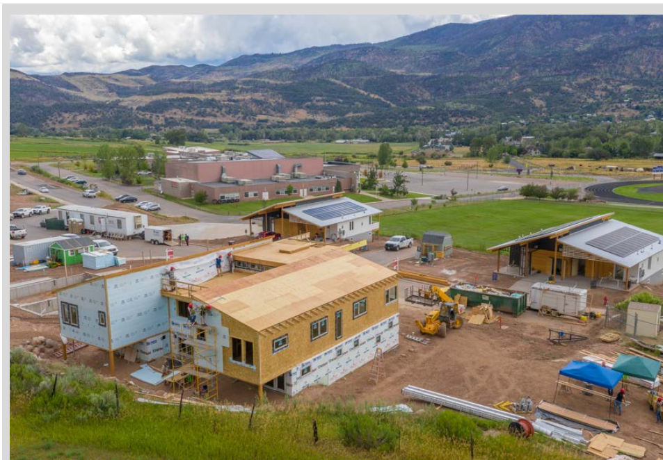
The Basalt Vista housing project, a collaboration between NREL and Holy Cross Energy, demonstrates the real-life applications of NREL's autonomous energy grid research. Photo by Josh Bauer, NREL
