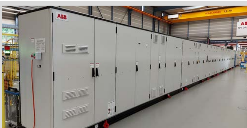
This converter assembly is a central component of the second controllable grid interface at the Flatirons Campus. When complete, it will help the U.S. electrical grid evolve by allowing a greater contribution from variable power generators, increased levels of energy storage, and smarter grid devices. Photo from ABB Group
