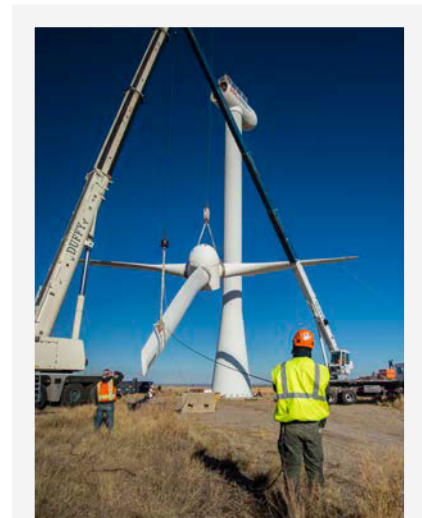
LandBOSSE helps users explore potential opportunities for reducing a wind project's total investment costs, including labor costs. Photo by Dennis Schroeder, NREL 53924
