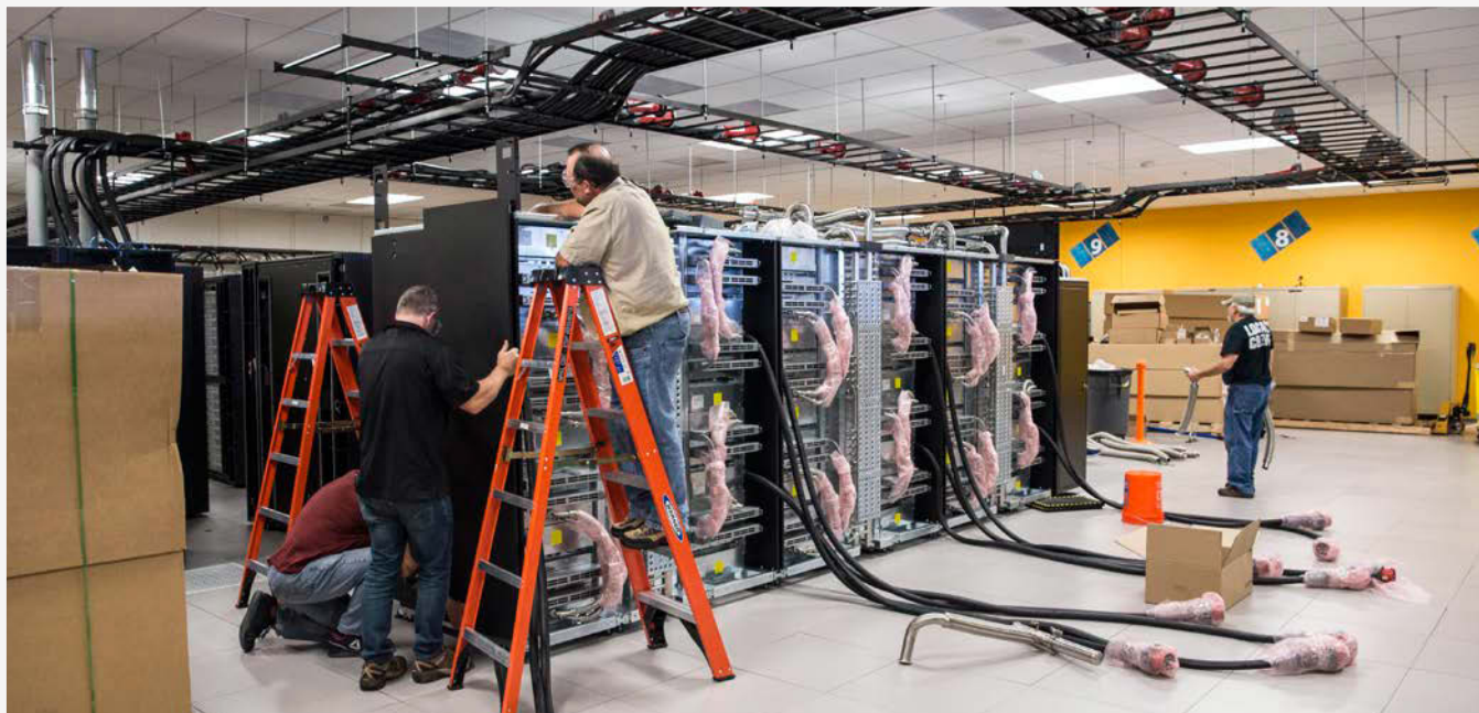
New software for new hardware. Existing weather models are becoming outdated because of their incompatibility with next-generation supercomputing architectures; therefore, ERF aims to address this. Photo by Dennis Schroeder, NREL 53208
