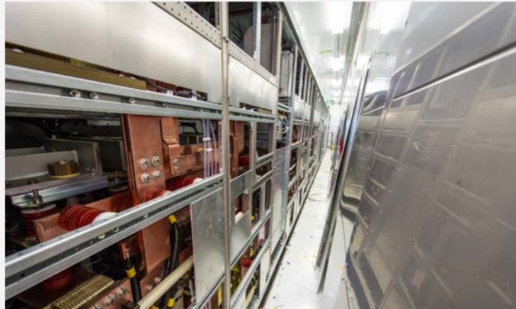
NREL's controllable grid interface (shown here), which is the centerpiece of the laboratory's grid integration testbed, was used to develop the world's first wind turbine impedance measurement system. Photo by Dennis Schroeder, NREL 27442
