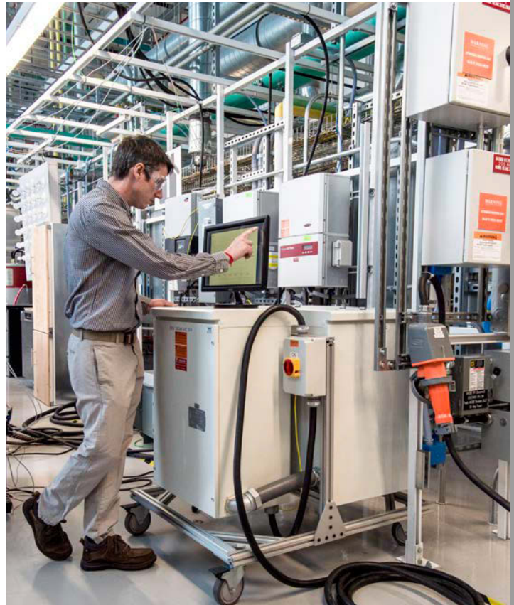
Researcher Scott Carmichael works with a home battery that integrates with a solar inverter and other controlled appliances as part of a home energy management system. Photo by Dennis Schroeder, NREL 45555
