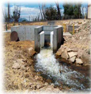
Figure 5. City of Cortez – 240 kW Water Treatment Plant Project. Photo courtesy of CWRPDA
