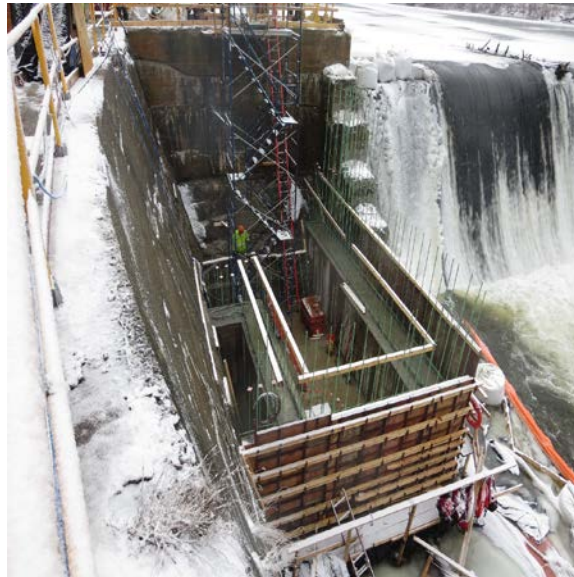
Figure 3. Glendale Dam Project – Minimum Flow Turbine Replacement. Photo courtesy of the MassCEC
