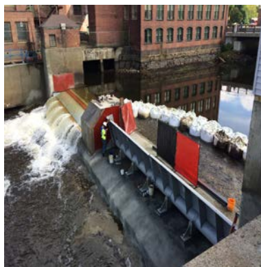
Figure 4. Mini-Watt Hydroelectric – 455 kW Project. Photo courtesy of the MassCEC
