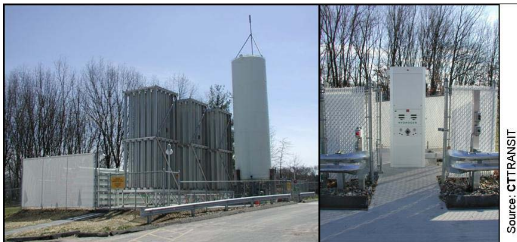
Figure D-2. Fueling facility (left) and dispenser (right) at UTC Power headquarters
