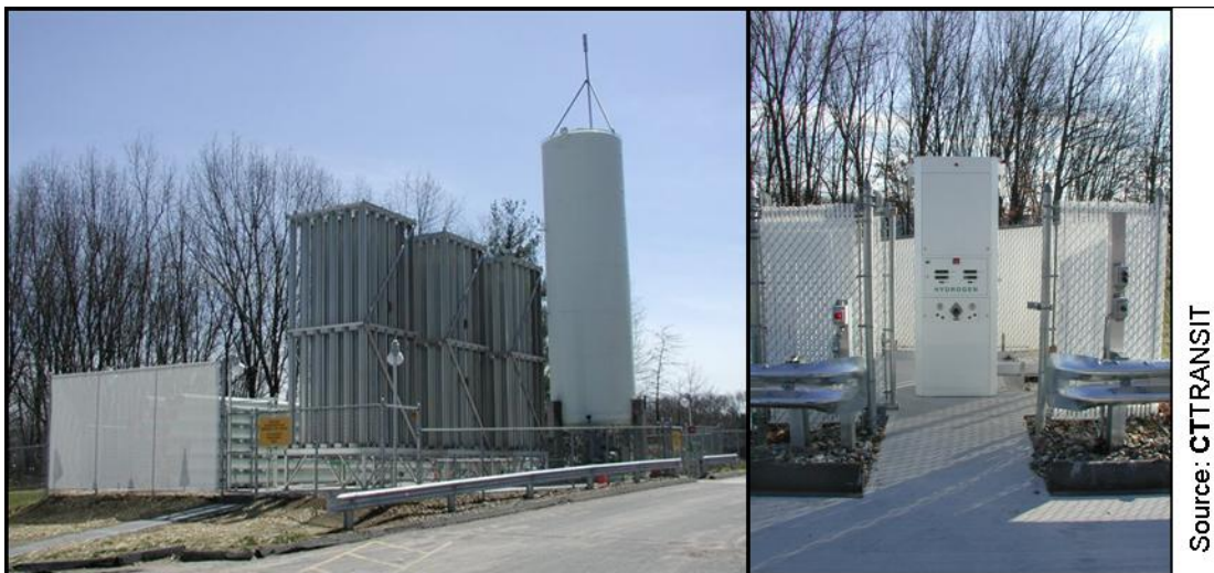
Figure 7. Fueling facility (left) and dispenser (right) at UTC Power headquarter
