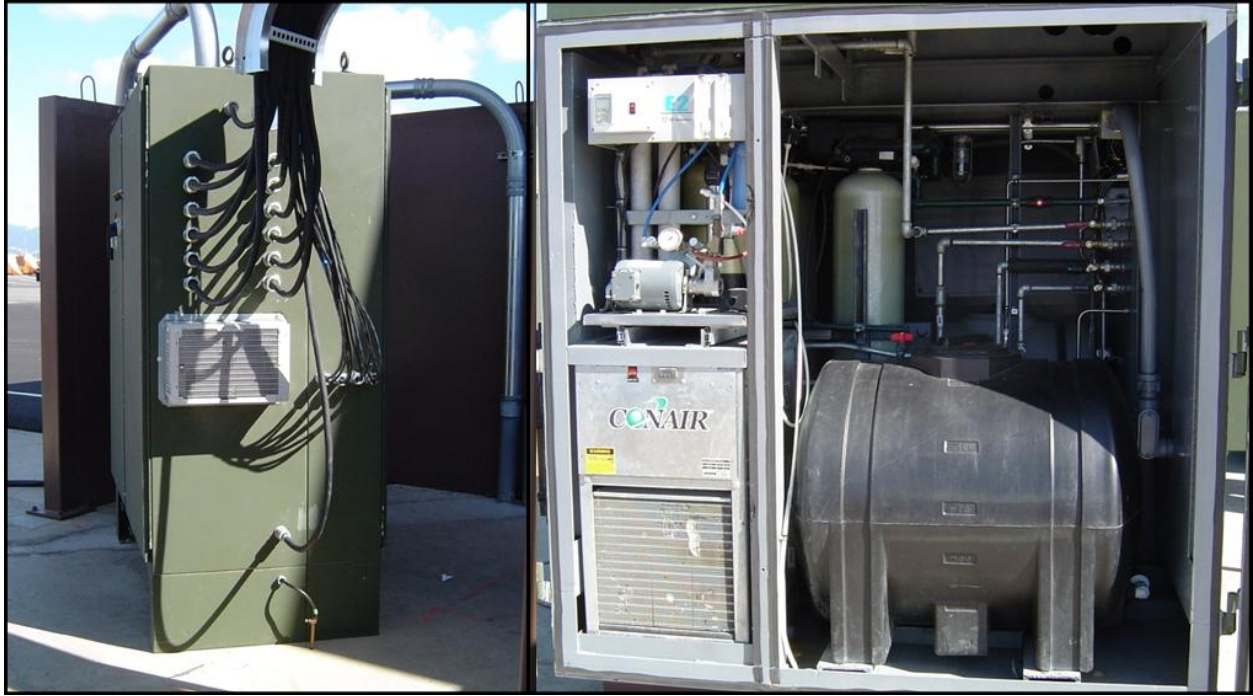
Figure 7. The power control unit (left) and water box (right)
