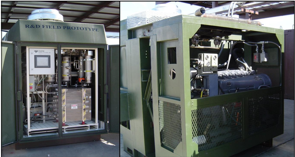
Figure 8. H 2 FP hybrid electrolyzer (left) and H 2 PM pressure management (right)
